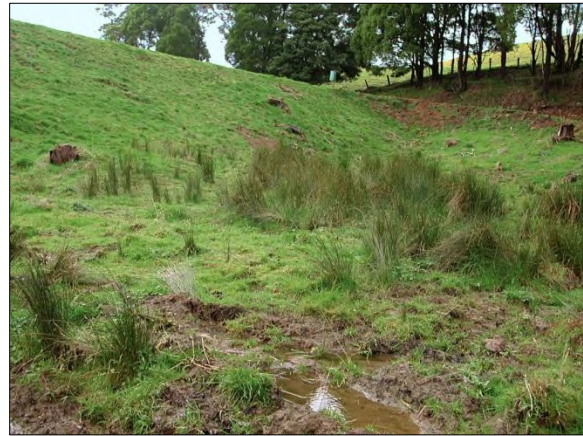
Earthen dam seepage
