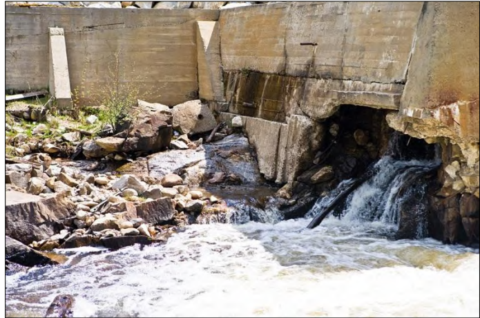
Piping flow through the dam as a result of dam concrete failure
